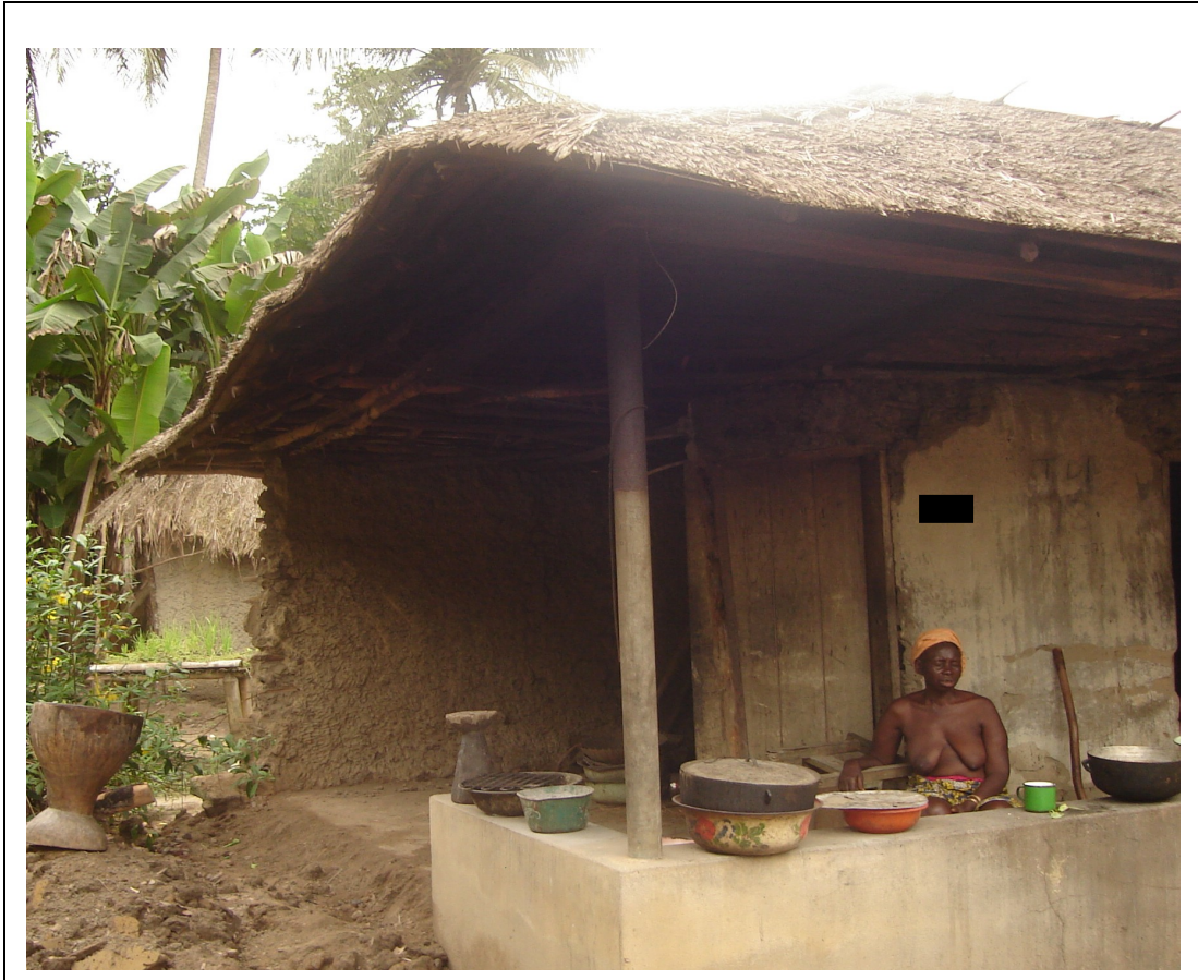
A collapsing house in Foida
